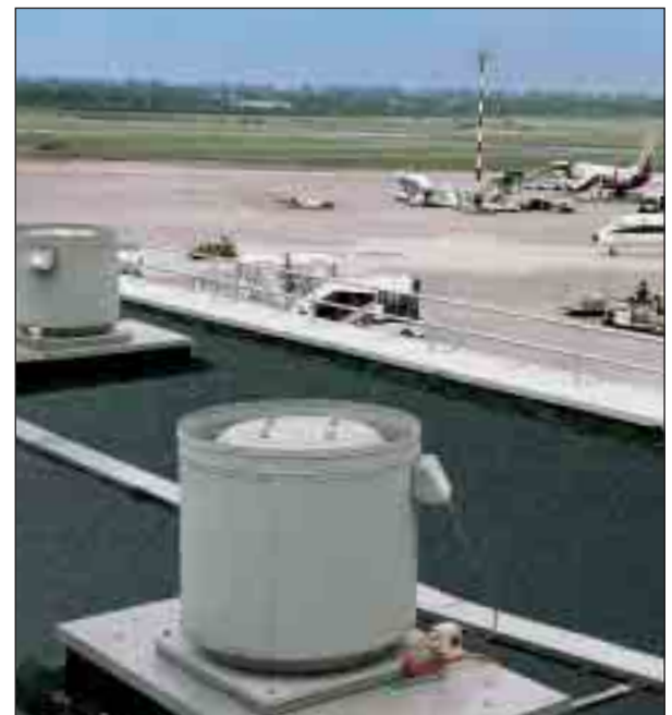
BVD smoke exhaust fans on a terminal roof at Düsseldorf Airport, gate C.
