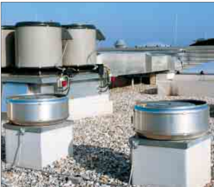
BVD roof-mounted smoke exhaust fans and DRV Minivent units on a building at the Franz-Josef-Strauß airport Munich
