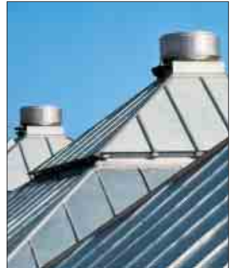
DRV roof units on the social services building of Maschinenfabrik Brose, Coburg
