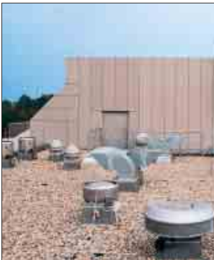
Various roof units on a technical building at the Free University of Berlin
