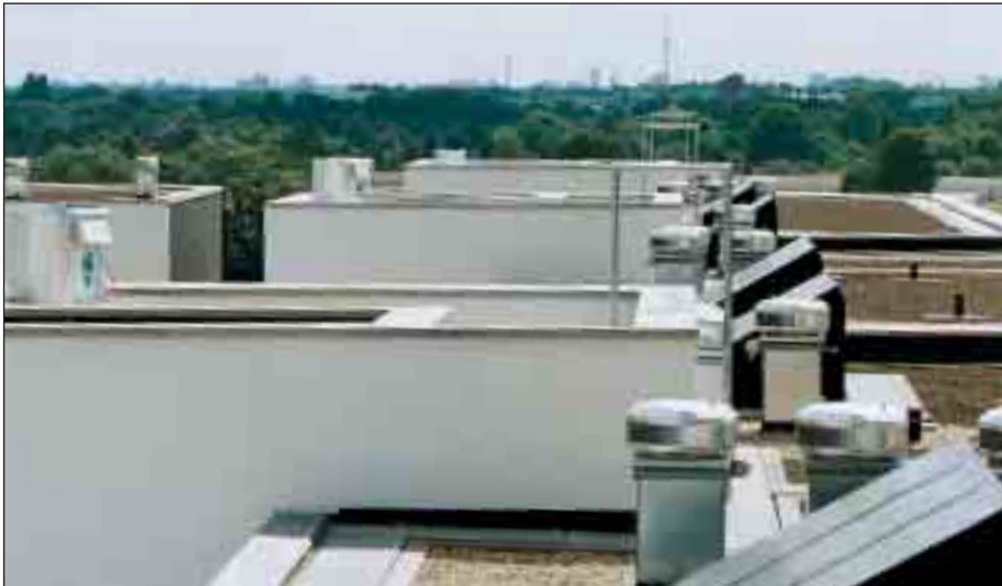
BVD roof-mounted smoke exhaust fans and DRH roof units with noise-damping base on a residential building complex (Wasserstadt, Berlin-Spandau)
