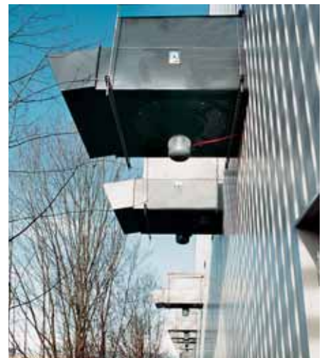
Wall-mounting smoke exhaust fans BVW-A Furniture store Unger, Wolfratshausen
