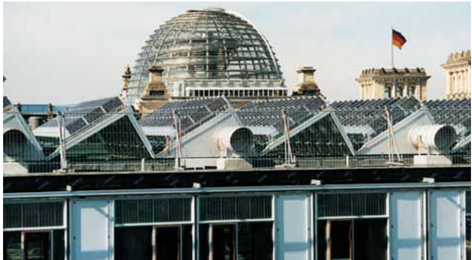
Axial smoke exhaust fan BVAX 12/56/800 for 300°C - 120 Min. with self-activating shutoff dampers (Dorotheen-Blöcke, Berlin)
