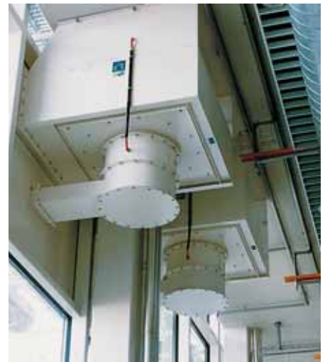
Wall-mounting smoke exhaust fans BVW-R Freight handling complex, Franz-Josef Strauss Airport, Munich
