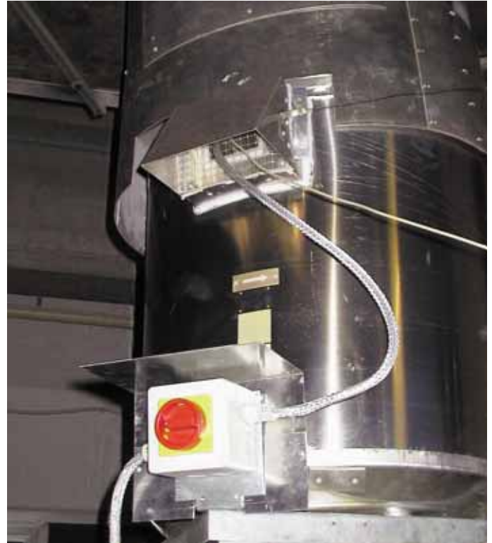
Heat-insulated repair switch, cooling air inlet nozzle
