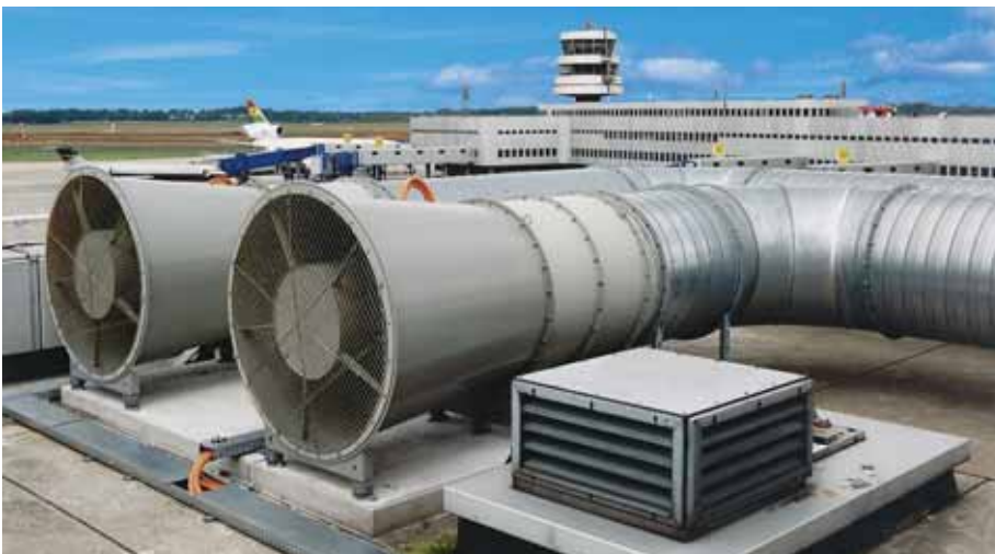
Axial smoke exhaust fans for 400°C–120 min. with outlet diffusers (Düsseldorf Airport, Terminal C)
