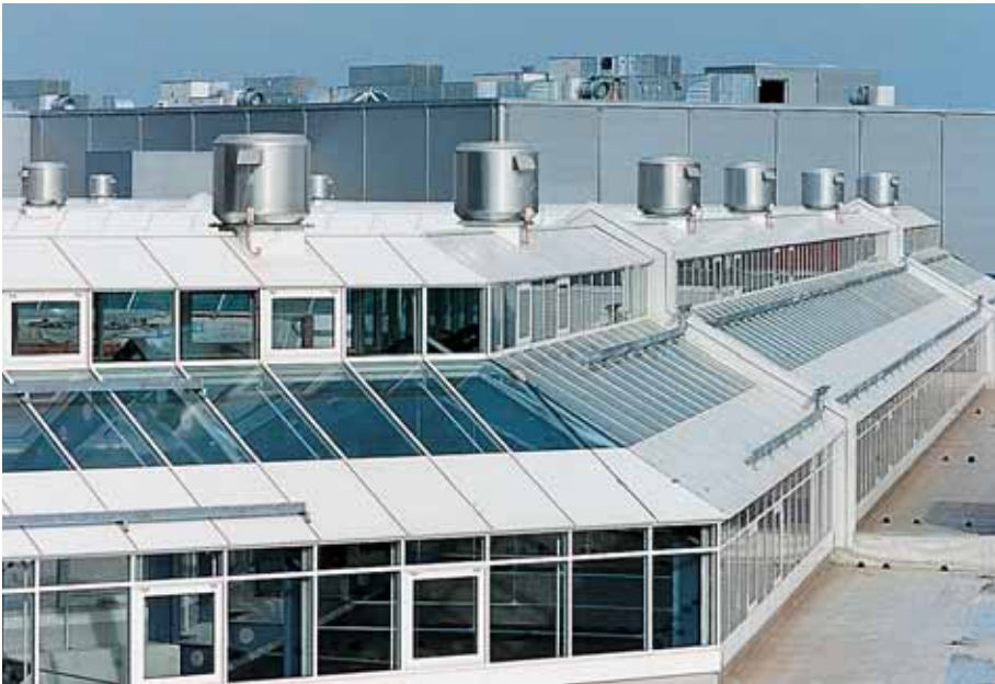
Roof-mounting smoke exhaust fans BVD and axial smoke-exhaust fans BVAXN (Leipzig, Paunsdorf shopping mall)
