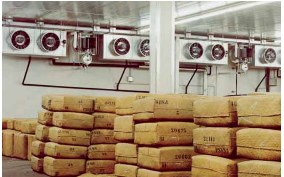
AXN 12/56/500 M-D axial-flow fans cooling a tobacco warehouse (Bremer Lagerhaus-Gesellschaft)
