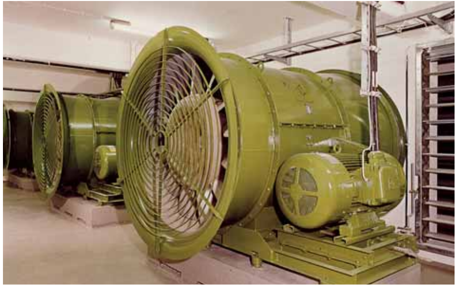
Type AXN 12/56/1600 R2 axial-flow fans in the air conditioning centre of a large office building (Hamburg-Mannheimer Versicherung)
